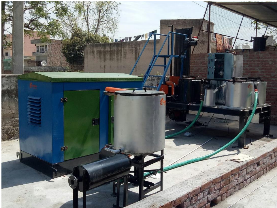
Figure 1: Typical small-scale gasification plant generating 5KW energy from the gasification of the waste.
